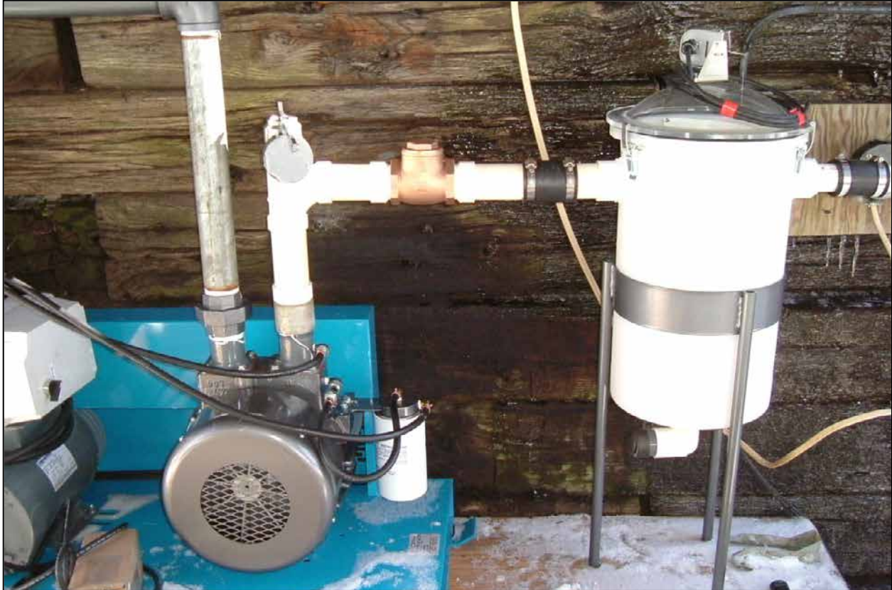
Vacuum pump and moisture trap set up outside the sugarhouse at the Arnot Forest
